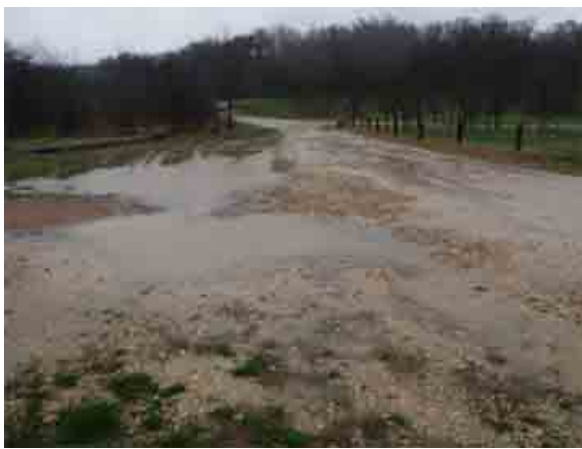
Diversion canal and culvert from CRR to LPNT will cross under the road just this side of the sign on the left side. Pond site is to the right. Foreground will be finished for parking.
